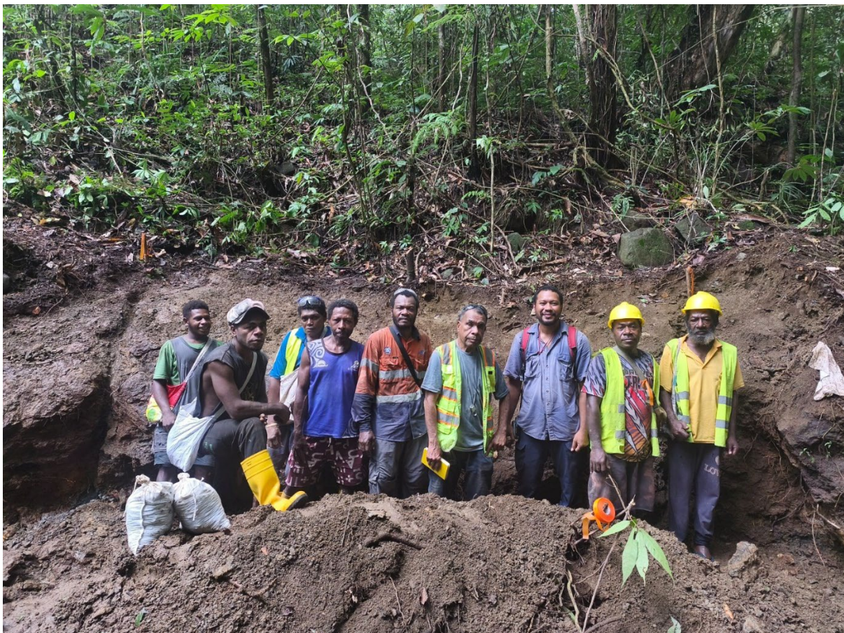
Figure 2: Trenching in progress at Agadul Prospect with Taruga's field team (Teatutai Sione – Principal Geologist 4 th from right).
