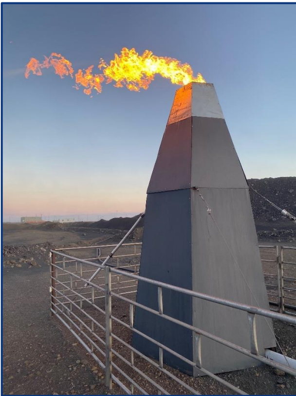
Existing Pilot Production wells in flare after commissioning new wells
