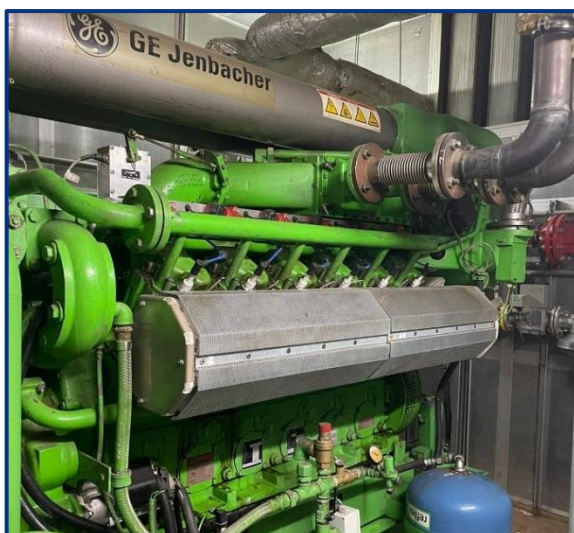
Typical small scale gas fired generator
