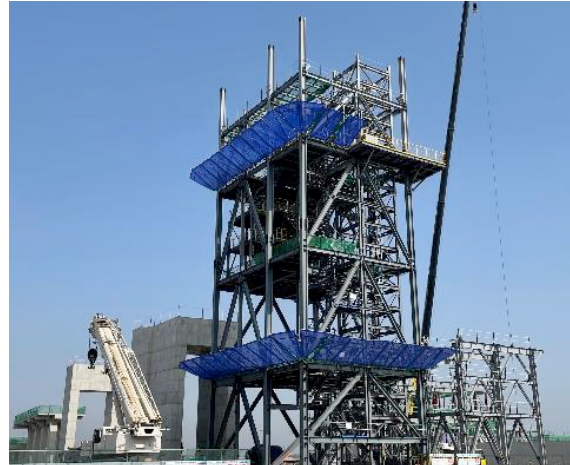
Acid roasting preheater
