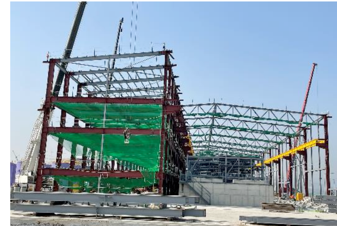
BPED (Bipolar Membrane Electro Dialysis) facility and electrical room
