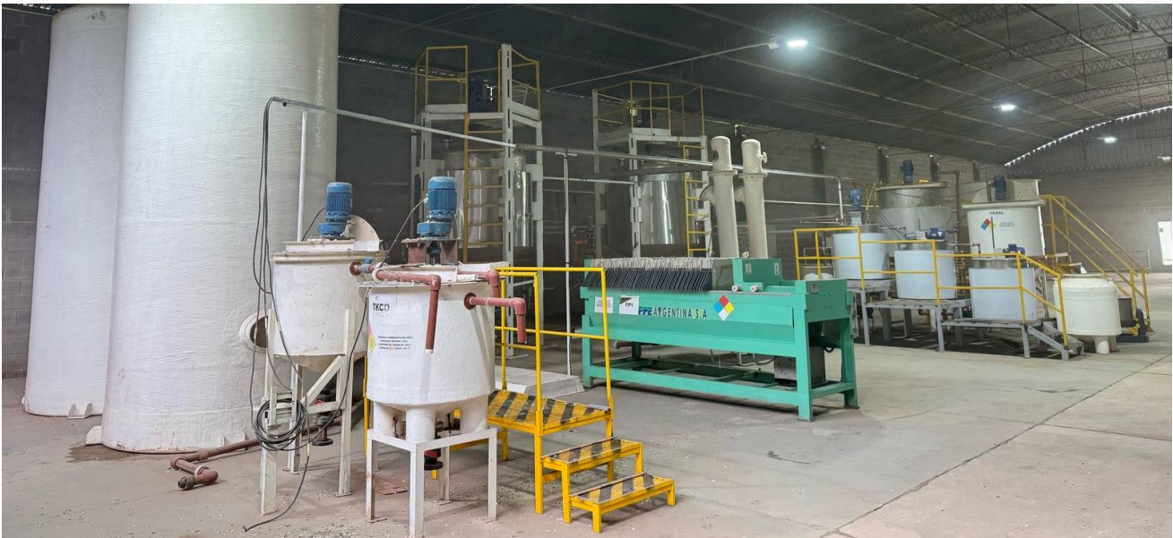
Figure 8: Pursuit's 250tpa Pilot Plant producing Lithium Carbonate in Salta, Argentina
