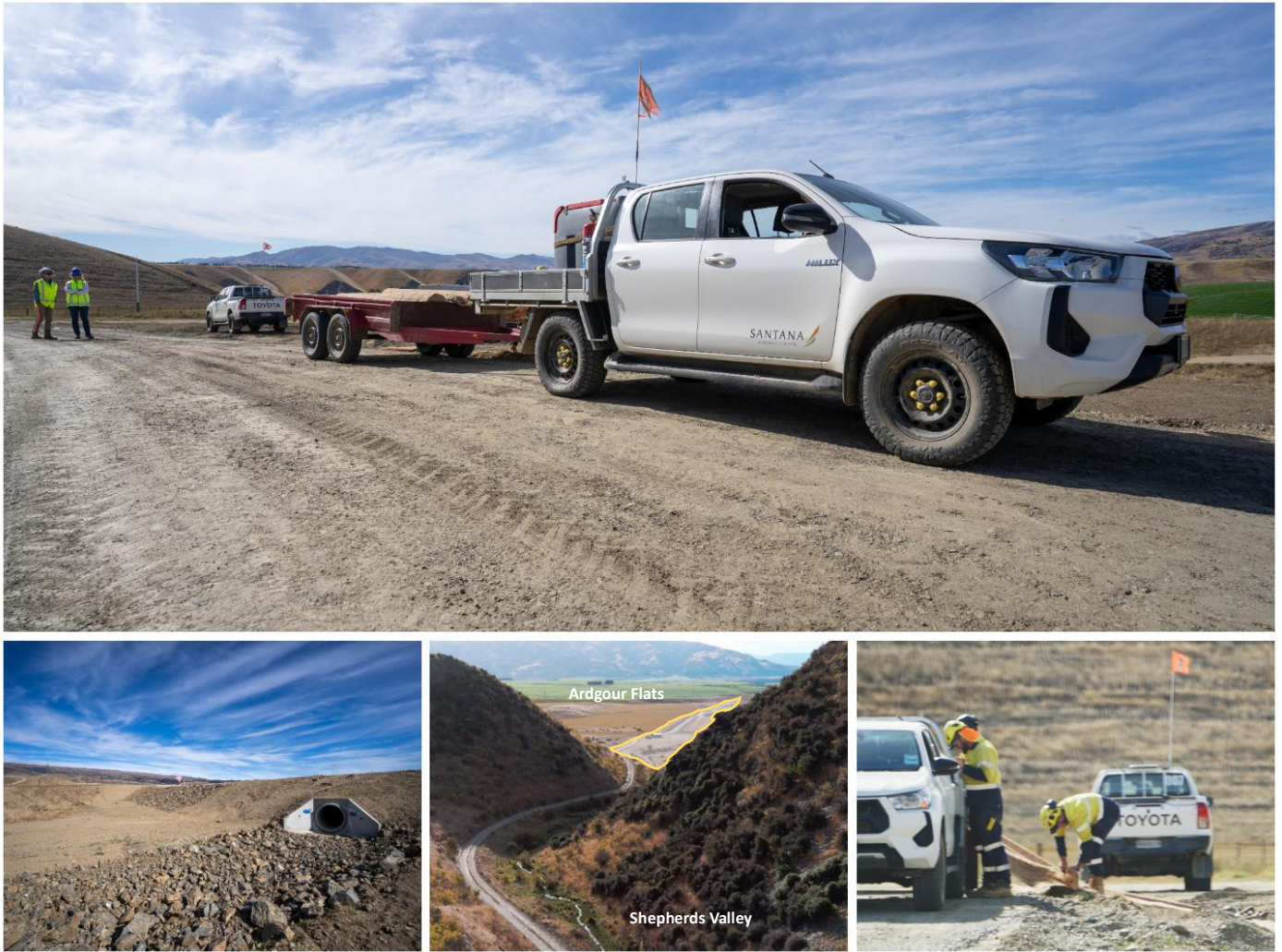
Figure 3. Santana construction teams executing permitted early works at the mine entrance on Ardgour Flats
