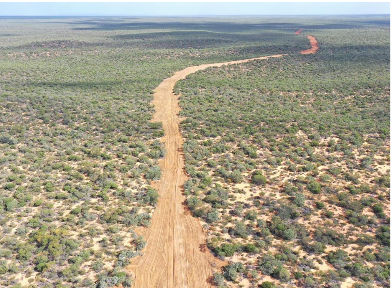
Figure 4 Coburn Project Clearing and Earthworks of the Main Site Access Road from the North West Coastal Highway
