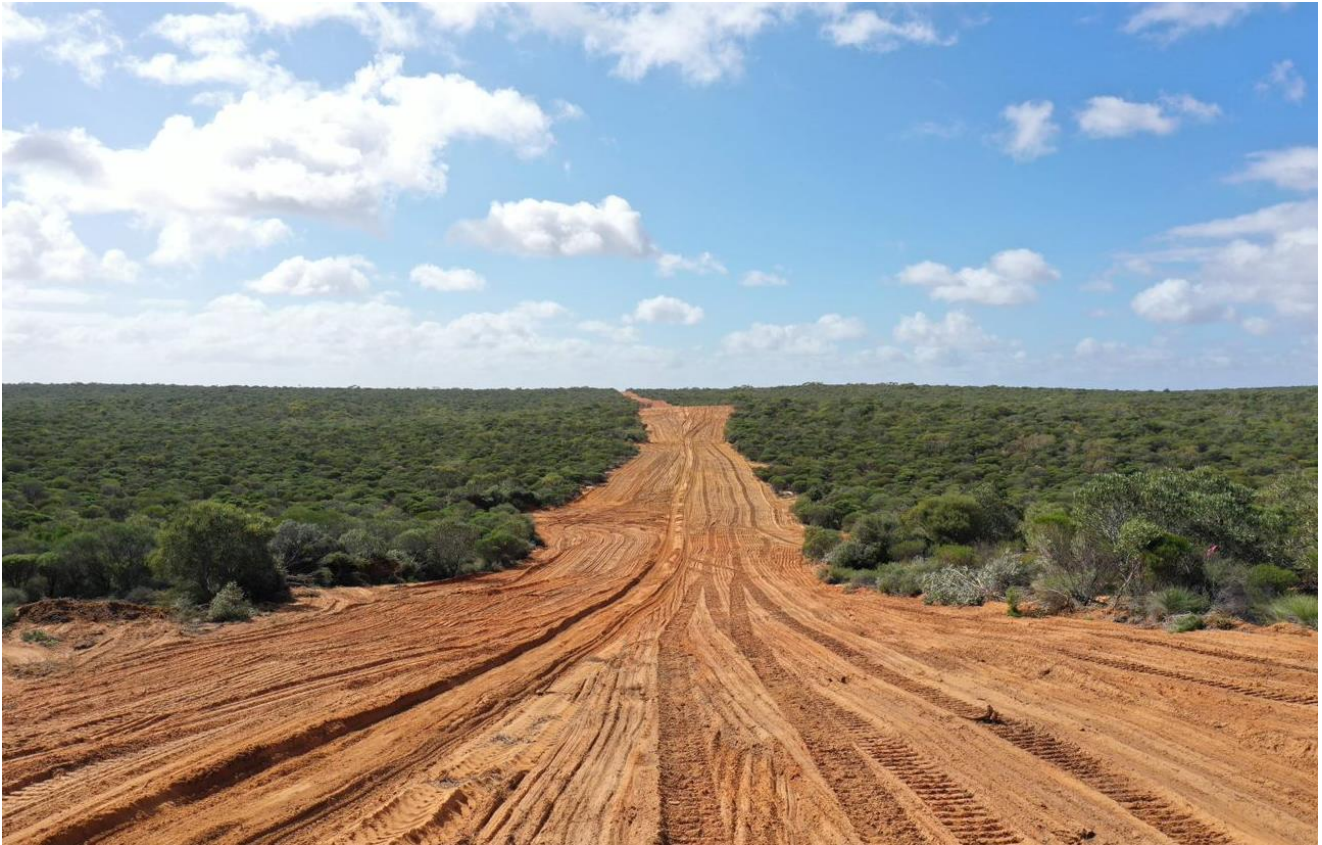
Figure 5 Coburn Project Clearing and Construction of the Main Site Access Road from the North West Coastal Highway
