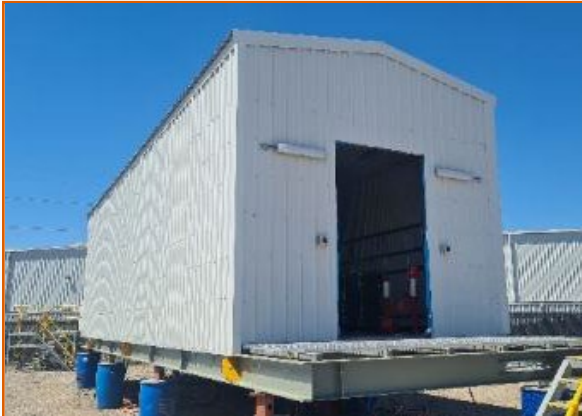
Electrical Switchroom Manufacture
