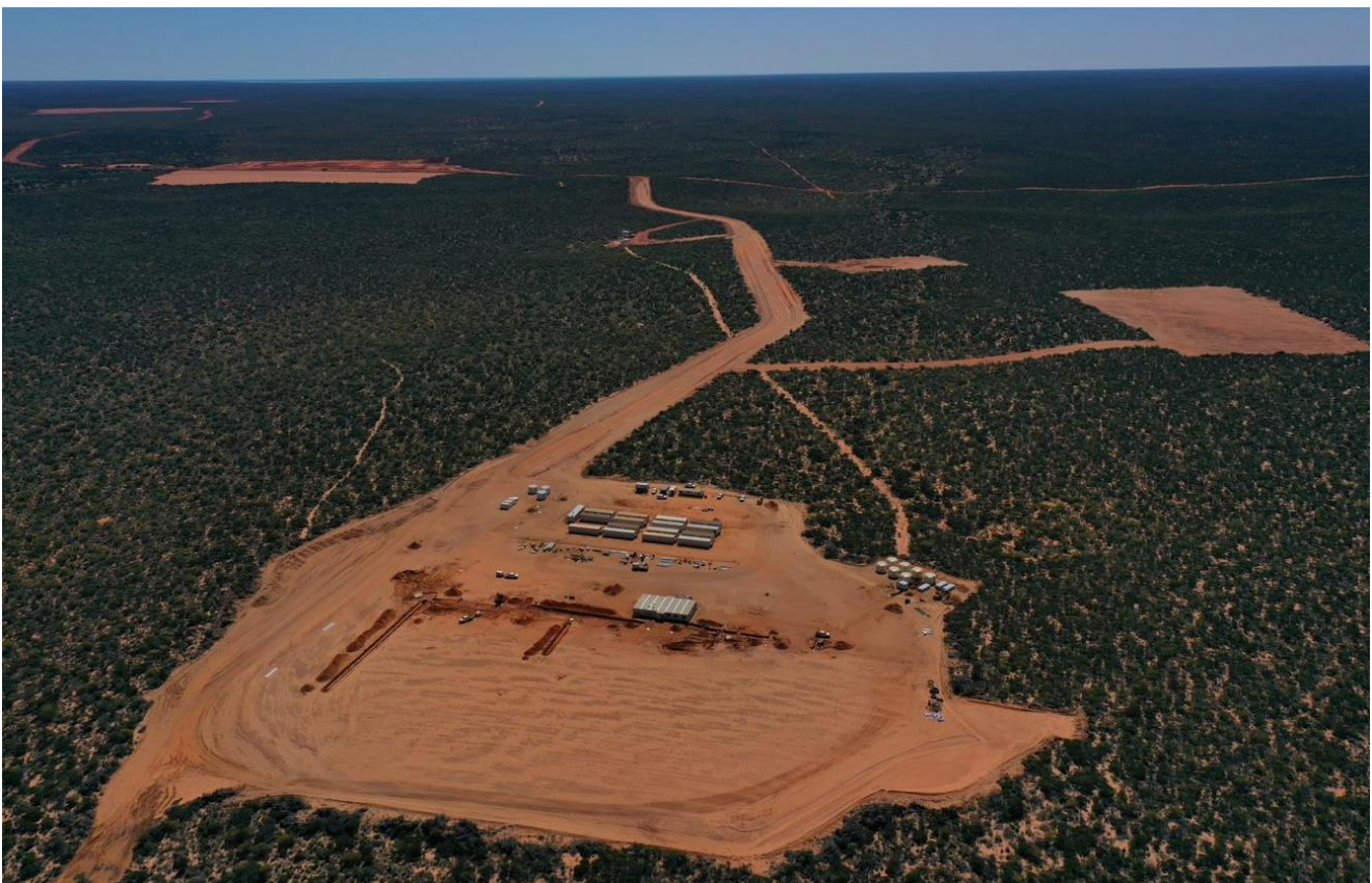
Figure 12 Earthworks Clearing Completed for all Infrastructure Areas including village, MSP, WCP and Bore Fields
