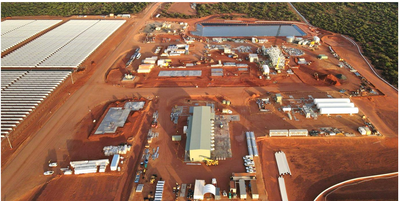
Figure 2 Coburn Project Mineral Separation Plant and Hybrid Power Station Area Progress Photos
