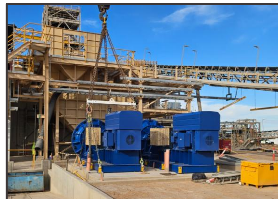
Ball mill discharge pumps
