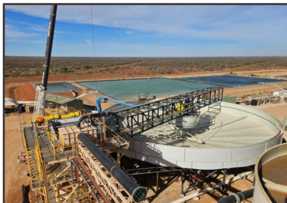
New tailings thickener
