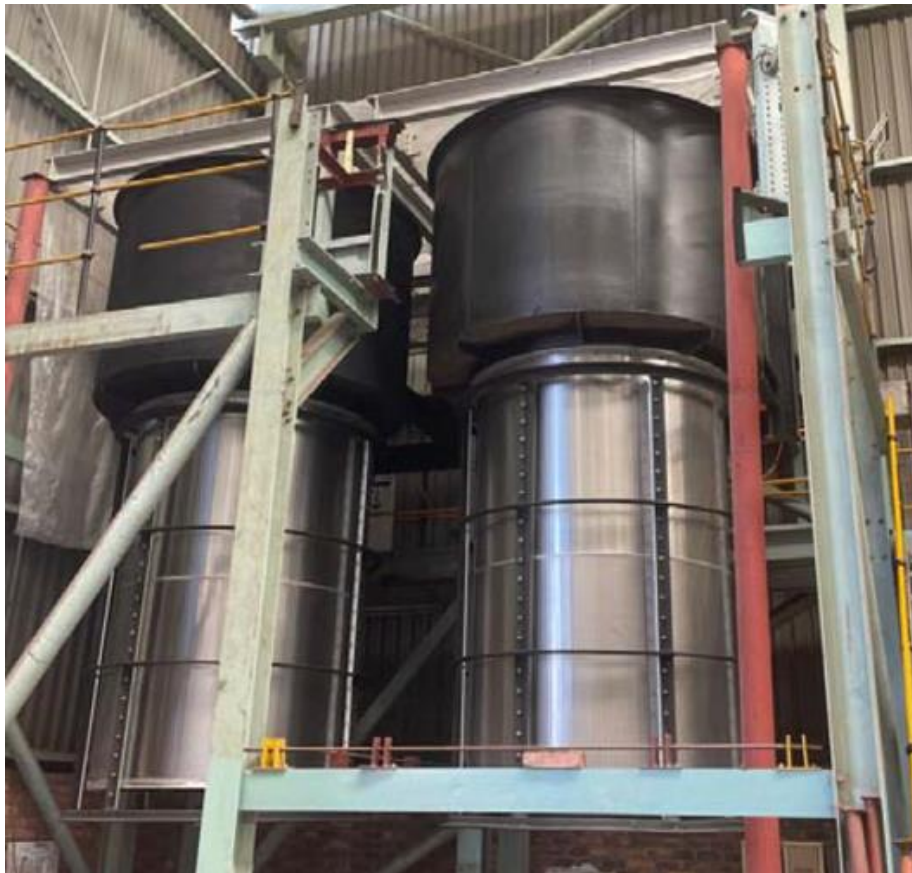
Figure 6: Intertank screens - Assembled and ready for Factory Acceptance Testing
