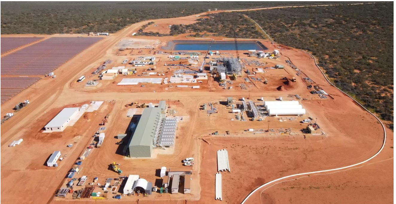
Figure 4 Coburn Project Mineral Separation Plant and Hybrid Power Station Area Progress Photos
