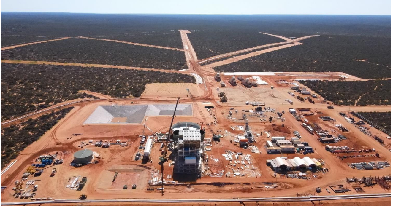
Figure 3 Coburn Project Wet Concentration Plant Area Progress Photos
