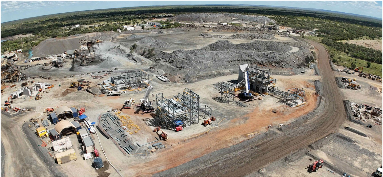
Photo 1: Current expansion work at Eloise. Ball mill raft concrete poured and backfilled (left), fine ore bin and emergency feeder (left-centre), screening and transfer area (front-centre) and primary crusher suspended slab concrete pour (right-centre).
