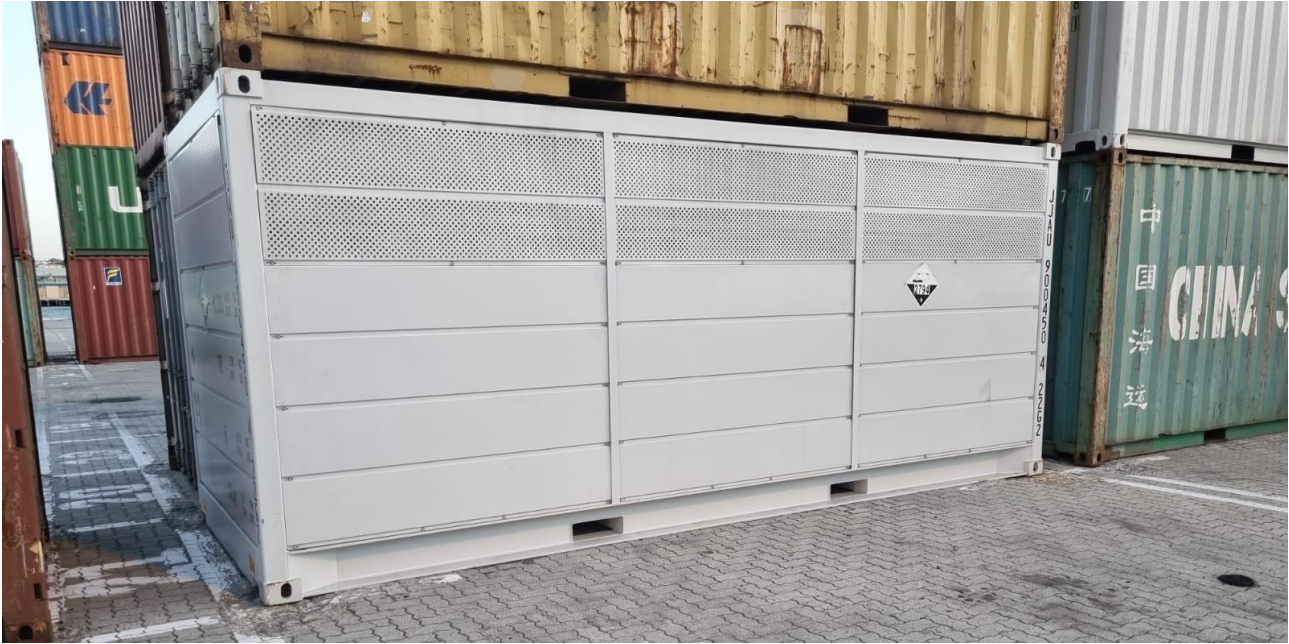
Figure 1 - Vanadium Flow Battery at Fremantle Port
