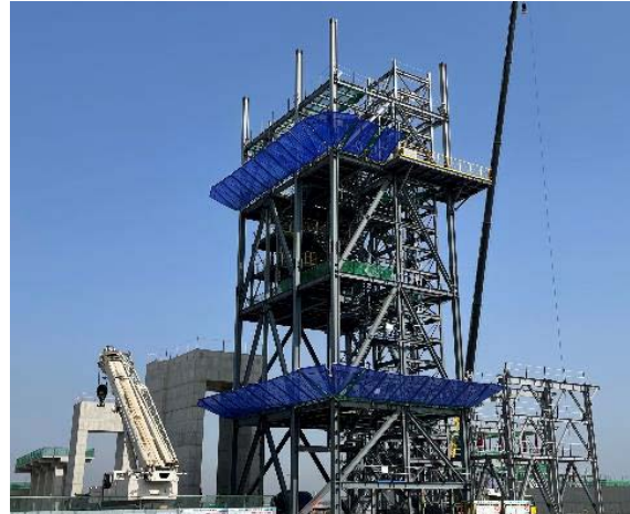
Acid roasting preheater
