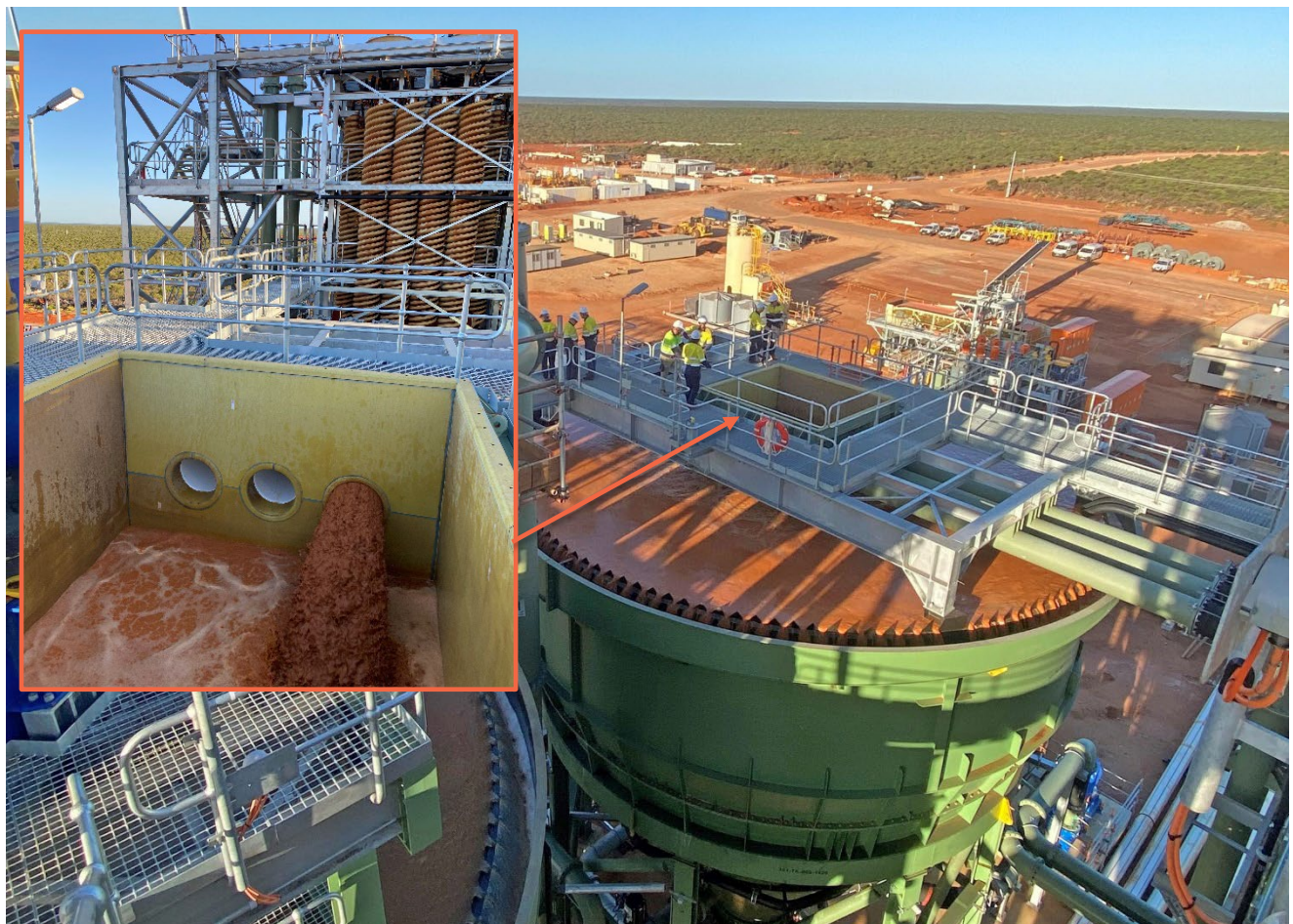
Figure 2 Coburn Project - Ore from the Mine Reporting to the Ore Receive Hopper at the Wet Concentration Plant
