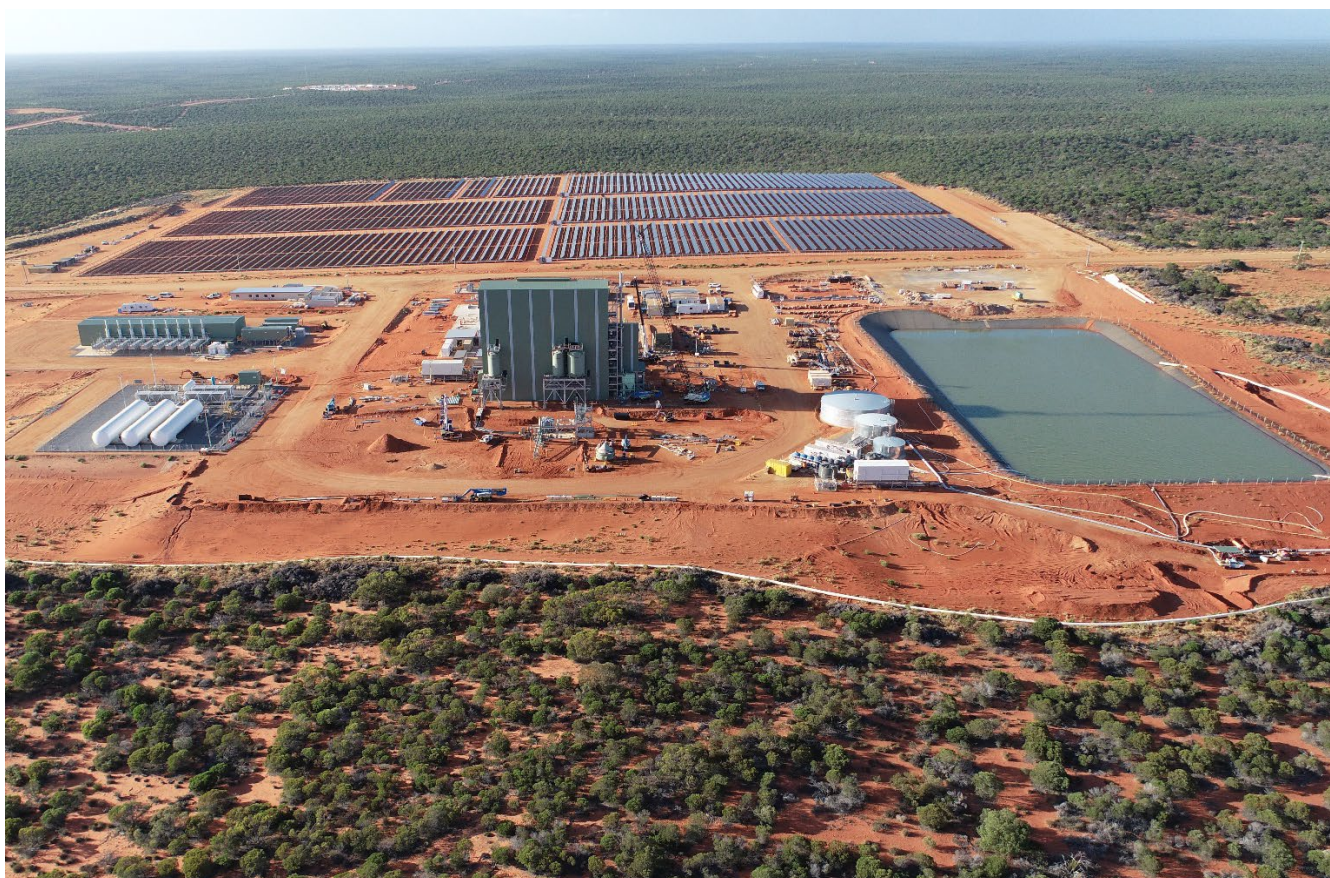
Figure 6 Construction of MSP and supporting infrastructure advancing in parallel with WCP commissioning
