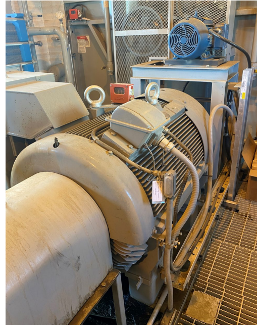
Bantry 2-29 600 hp Compressor recently replaced
