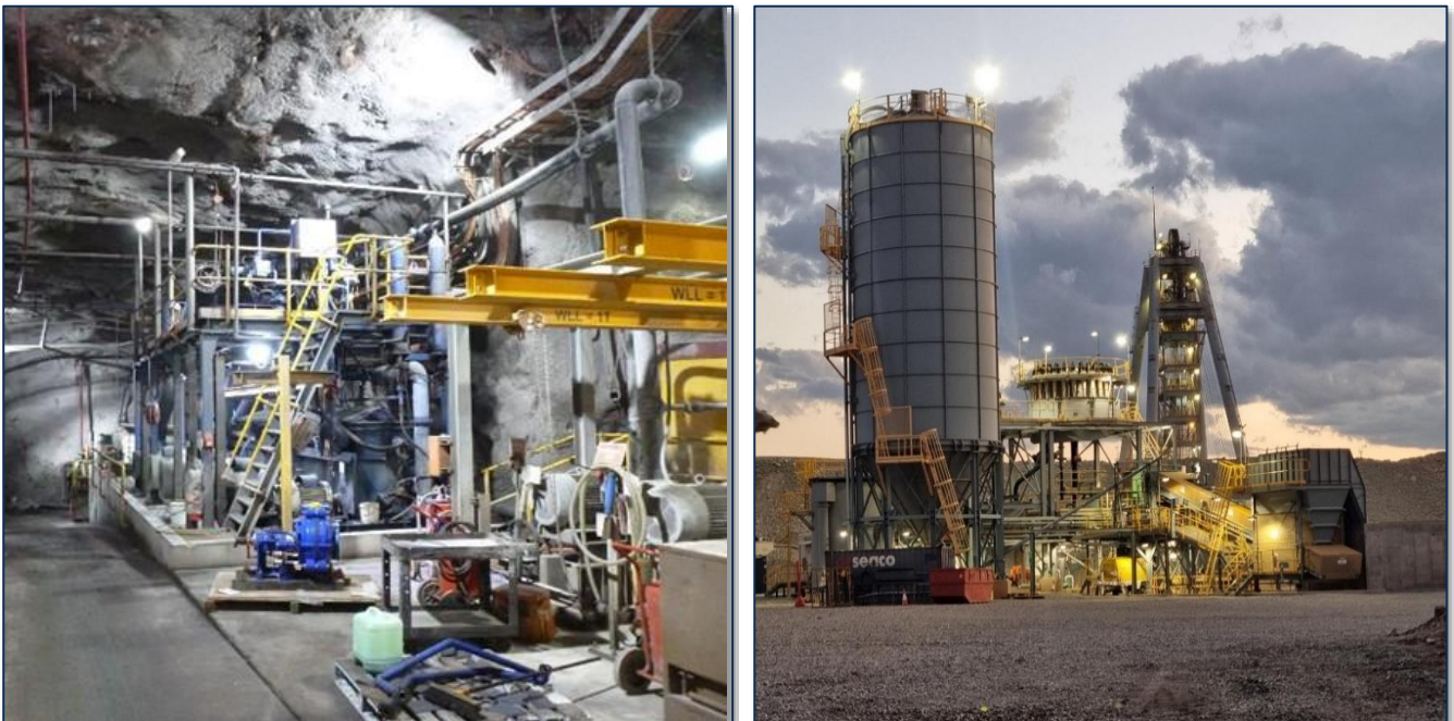
Figure 5: MDU water pumping station (left) and paste plant (right foreground)
