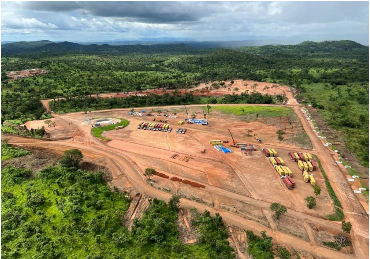
Photo 2. Aerial view of commencement of mobilisation of 1,500-person temporary construction camp in Beyla to service the CTG Simandou Infrastructure Project underway, located approximately 100km south of the Simandou
