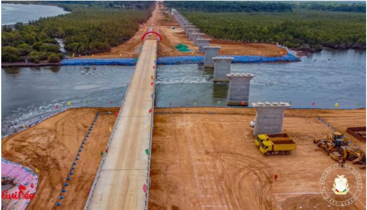
Photo 1. Newly constructed traffic bridge over the Mamkudu River in Guinea officially opened in May 2023 with pylons for the railway bridge alongside (courtesy of Government of Guinea).
