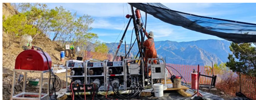
Figure 1. Diamond rig set up at the site of Advance's first drill hole at the Gavilanes Project in Durango, Mexico.
