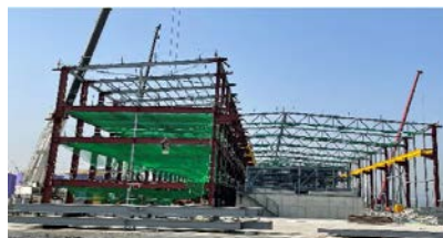
Figure 3: BPED and Electrical Control Room
