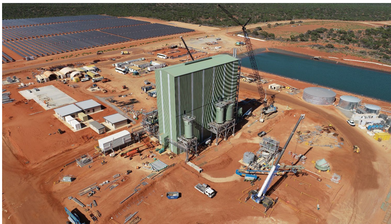
Figure 4 Construction of MSP and supporting infrastructure advancing in parallel with WCP commissioning
