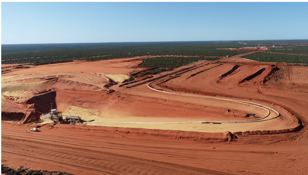
Figure 2 Pre-production development of Coburn's open pit mine is complete with all Dozer Mining Units connected
