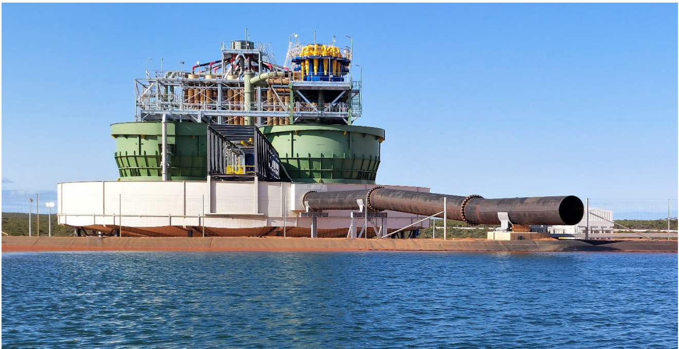
Figure 1 Final construction verification, water commissioning and sequence testing of Coburn's Wet Concentration Plant underway
