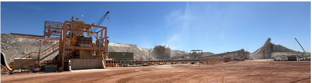
Figure 3: Crusher CV01 transfer box to CV03 conveyor extension to existing plant
