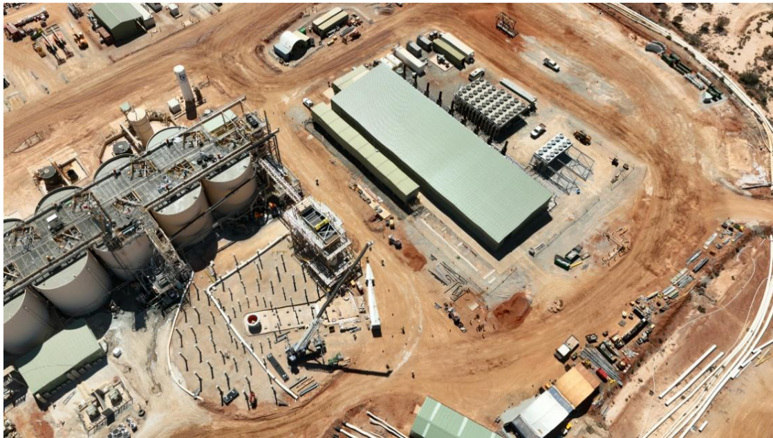
Figure 2: Stage 1 wet plant upgrade complete with 4 new CIL tanks online. Stage 2 works including a tailings thickener and powerhouse extension progressing well
