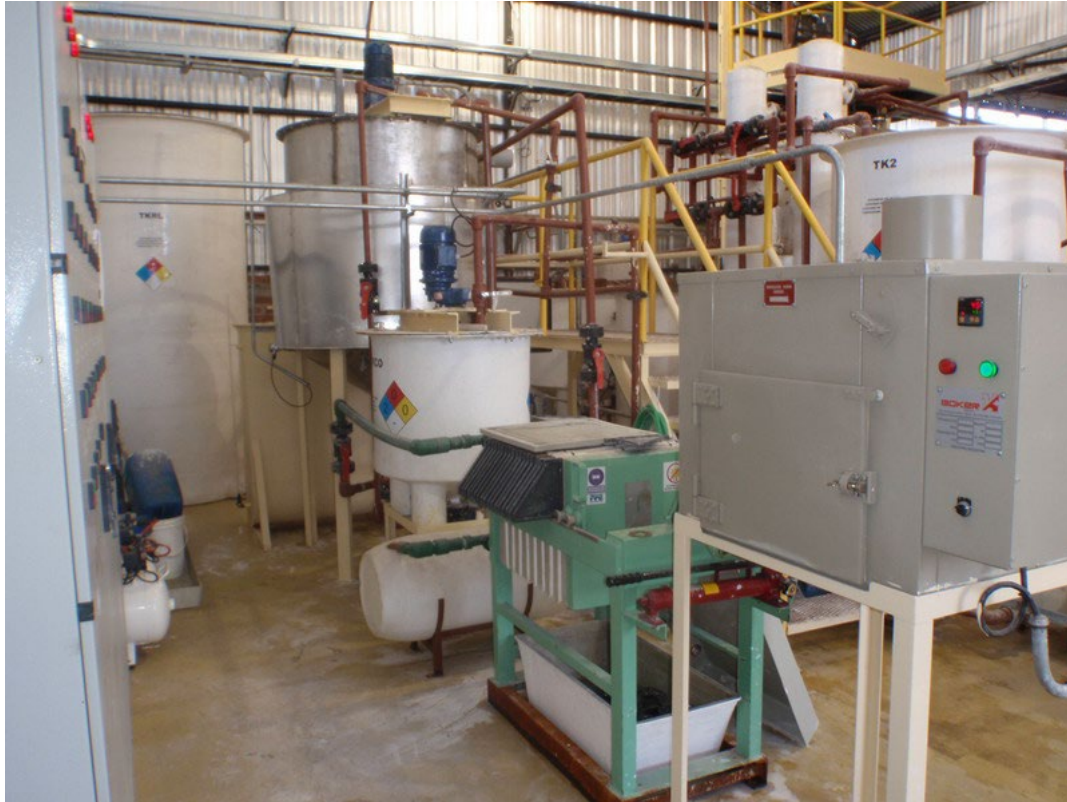
Figure 3 – Lithium Carbonate Pilot Plant
