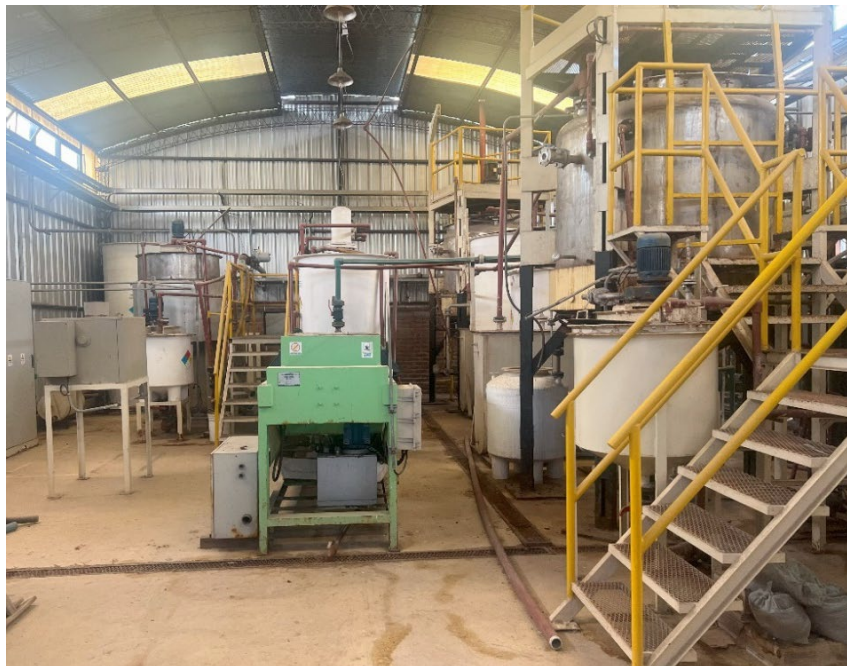
Figure 1 – Pilot Plant during site visit March 2023
