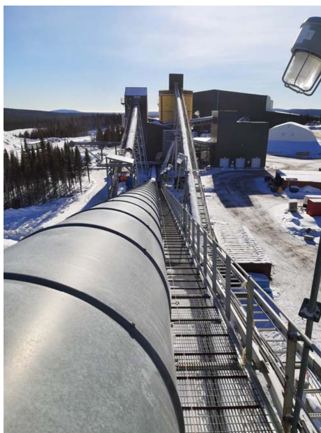
Crushing infrastructure and main conveyors, NAL
