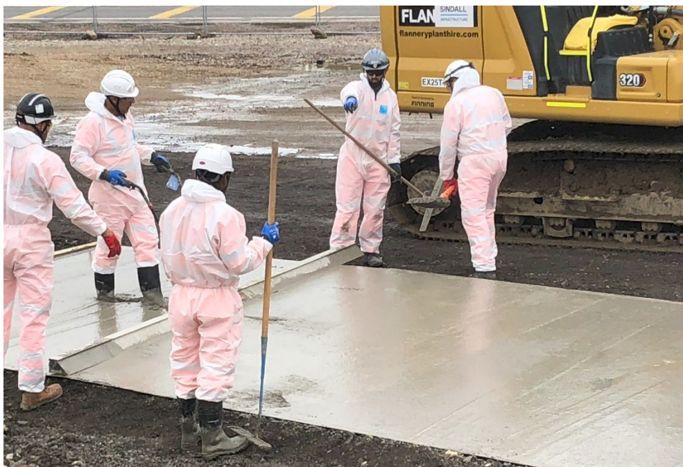
Figure 1: Graphene-enhanced cement application at major UK infrastructure project, delivered by Morgan Sindall Infrastructure.
