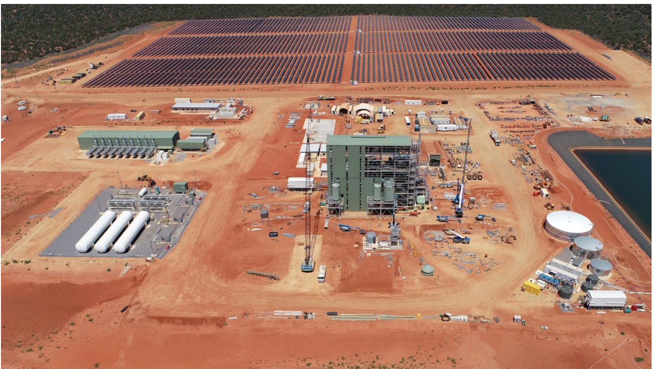
Figure 2 Construction of MSP and supporting infrastructure advancing in parallel with WCP commissioning
