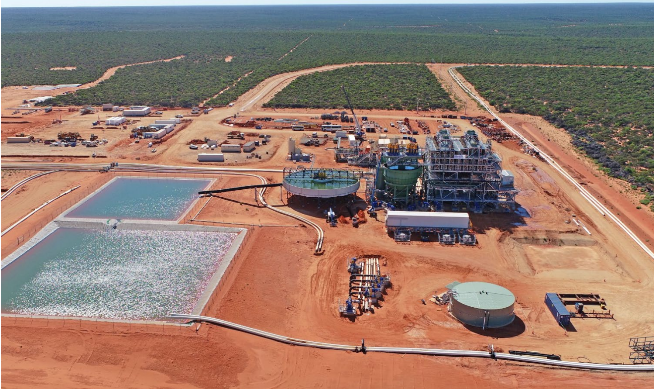
Figure 1 Final construction verification, water commissioning and sequence testing of Coburn's Wet Concentration Plant underway
