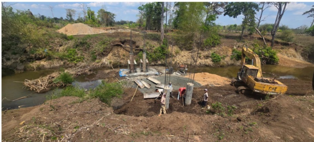
Figure 24 | Commencement of works on new community bridge across the O’Pung Toul River
