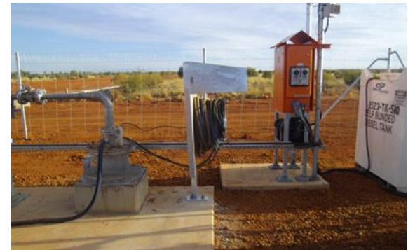
Image: Typical Bore Field Pump Station
