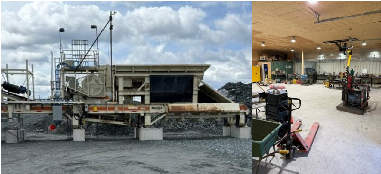
Figure 5: New crusher footings in place and inside of new mill maintenance workshop
