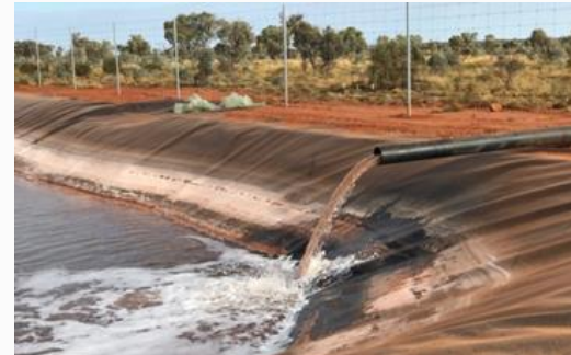
Image: Typical HDPE lined Water Pond
