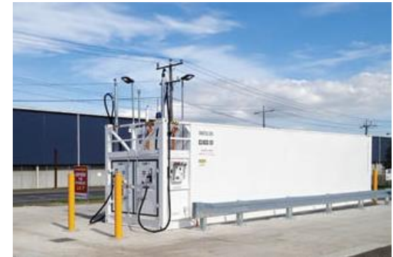
Image: Example of self-bunded diesel storage facility
