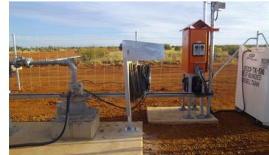
Image: Typical Borefield Pump Station Installation
