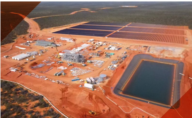
FIGURE 5: CONSTRUCTION OF COBURN'S HYBRID POWER STATION, MSP AND SUPPORTING INFRASTRUCTURE ADVANCING STRONGLY IN PARALLEL WITH WCP
